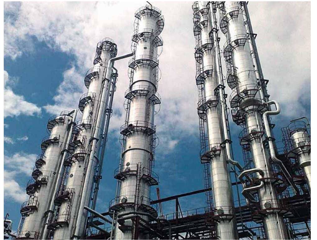
A total of 13 columns were built for the extensions to butadiene production at the Kralupy plant.
