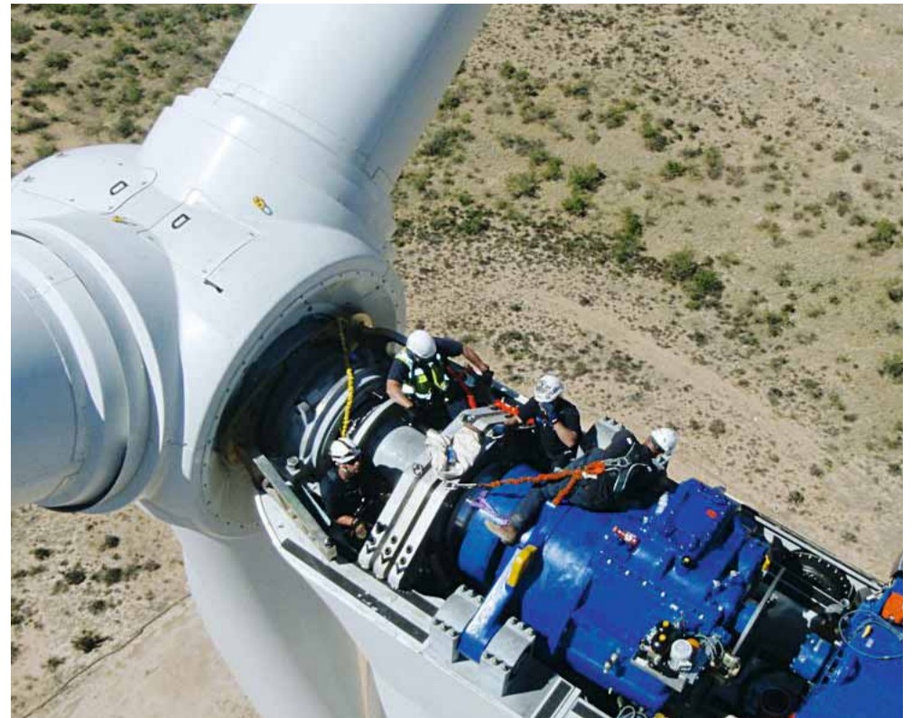
The specialists from BIS Salamis Inc. climb up a ladder to enter the nacelle. High temperatures can impede work in the summer months in particular.
