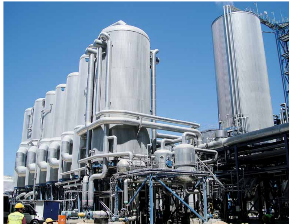
The new vaporisation system was insulated with stone wool and stainless steel panelling.
