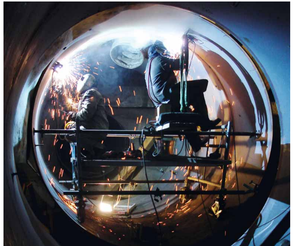
There was very little space for working on either side of the new pipe due to its wider diameter. Because of this, the welding had to be performed inside the pipe. Welding smoke was extracted using special hoses.
