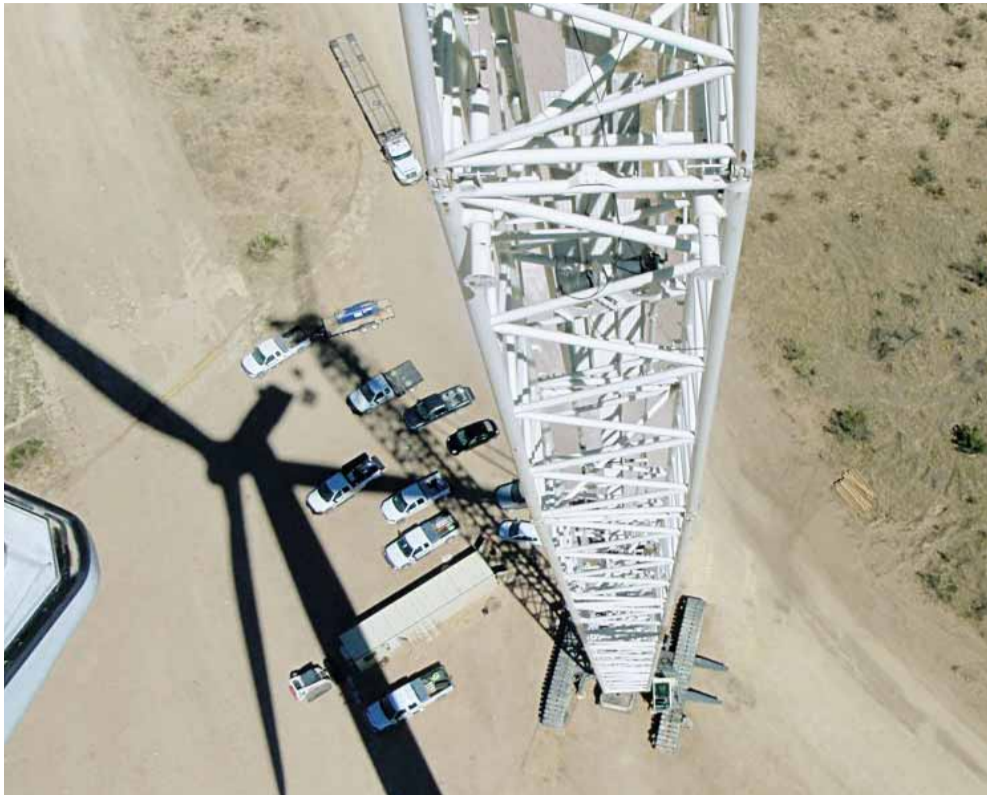
Some wind power systems have a height of over 90 metres. BIS Salamis Inc. uses one of the world's largest mobile cranes to replace the 20 ton transmission.
