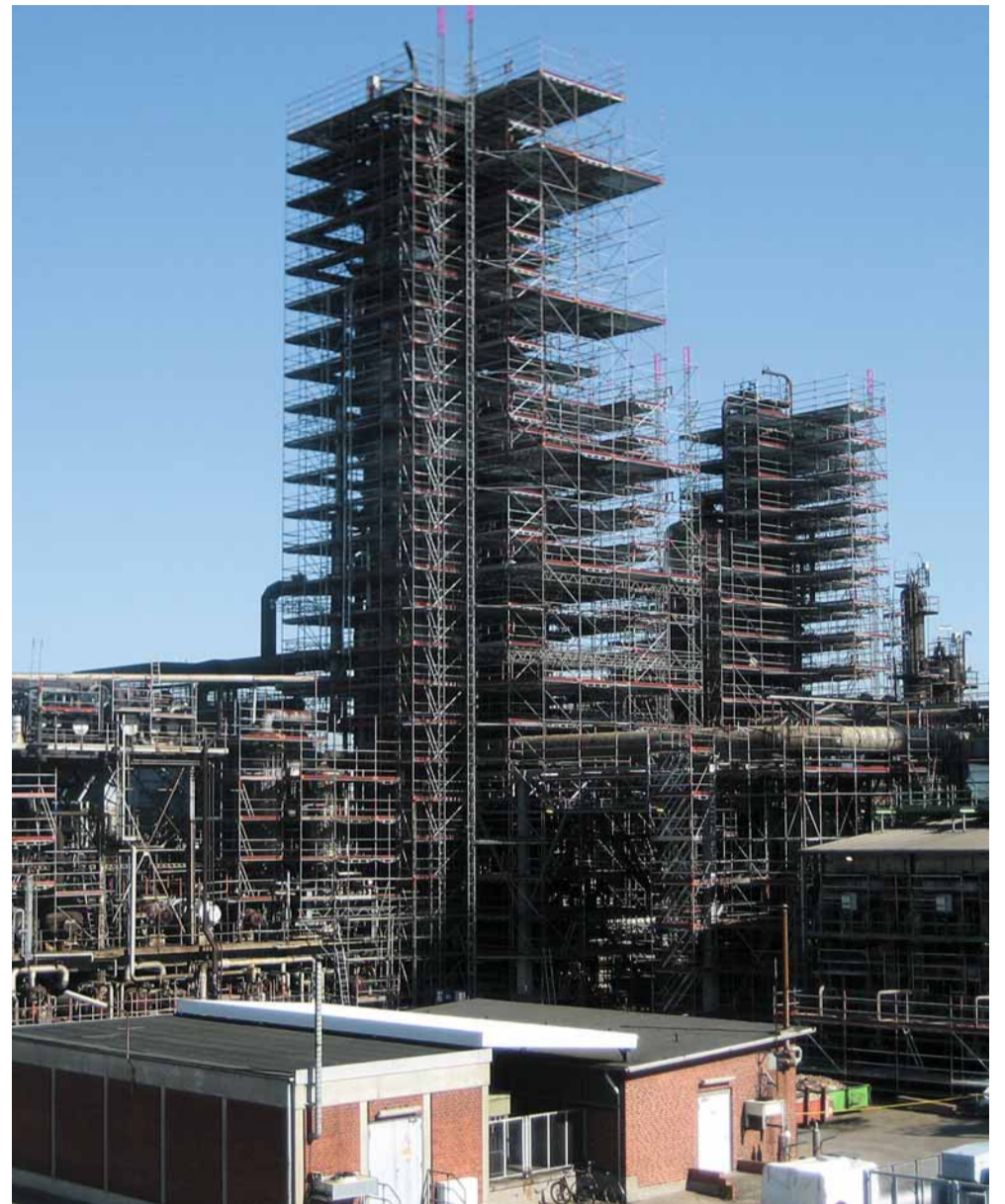
Scaffolding was necessary for four columns during the second major turnaround in the northern part of the refinery. 16,000 m 3 of scaffolding was required for a single column.
