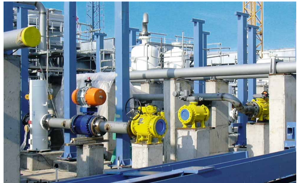
The piping fitted to the new gas accumulator is designed to withstand extremely high pressure of between 120 and 160 bar. This called for careful inspection of the welding seams.
