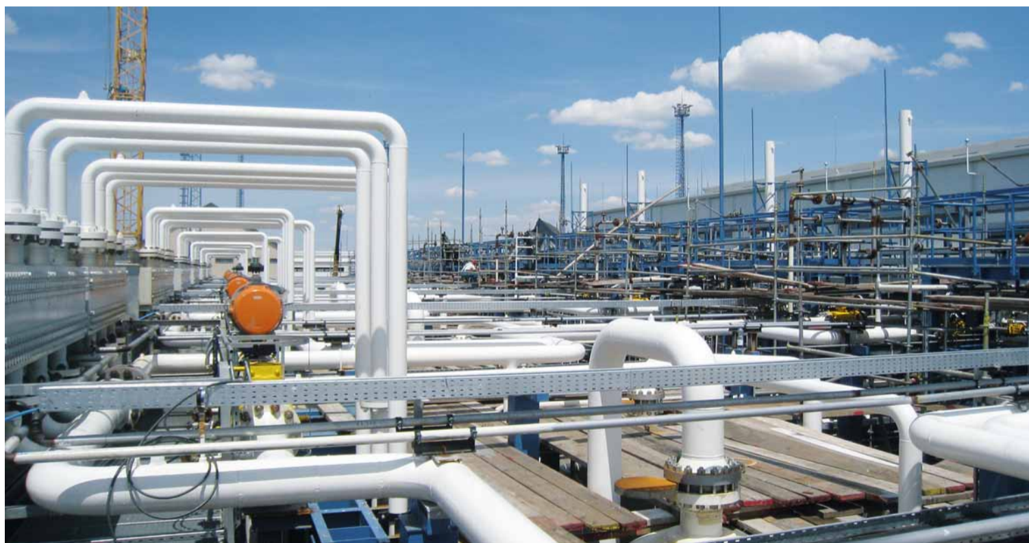
Surface and subterranean high-pressure piping of a total volume of 260 tons was required for the "Szőreg-1" gas accumulator. BIS Hungary prefabricated around 60 percent of this at its workshop in Tiszaújváros.
