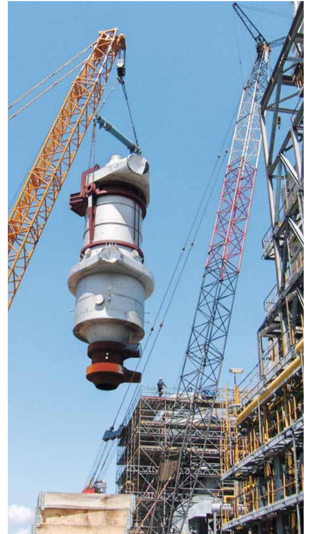
The 330-t styrene reactor requires the use of a special crane at the BASF plant in Antwerp.
