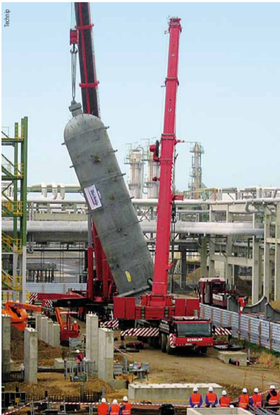
The reactor, measuring almost 20 metres in length and weighing 115 tons, travelled about 5,000 kilometers from France before arriving at Leuna.
