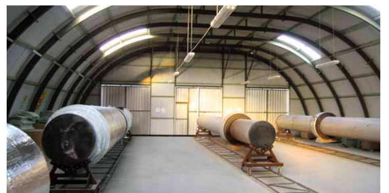
Pipeline construction and insulation activities in southern France require shelter from the Mistral.
