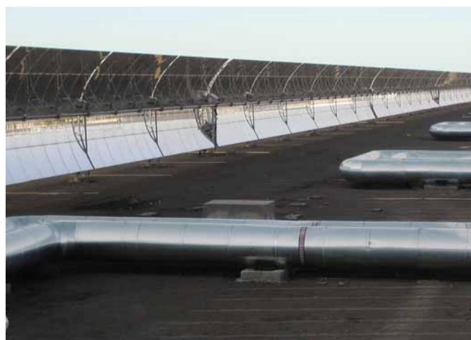
The Spanish and Polish BIS affiliates were responsible for insulating the large-diameter pipes during the construction of Andasol 1.
