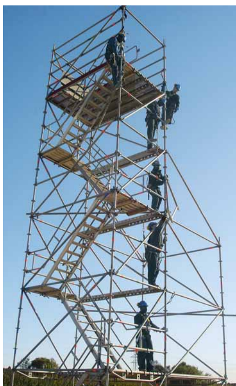
Worker safety on scaffolding is a top priority for BIS. This is something customers appreciate.
