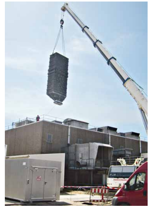
The operation to lift the 35-ton recuperator went smoothly, as did the installation of the new eleven-metre exhaust terminal.
