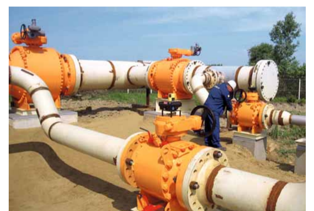
The pipelines and fittings for the new compressors are impressive in their dimensions.
